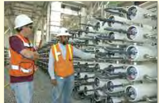
Photo courtesy of Orange County Water District
