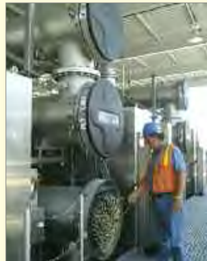
Photo courtesy of Orange County Water District
