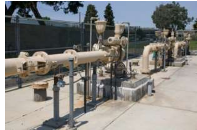
Typical injection well - OCWD
