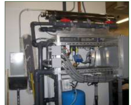
Recycling equipment, Valentine Engineering
